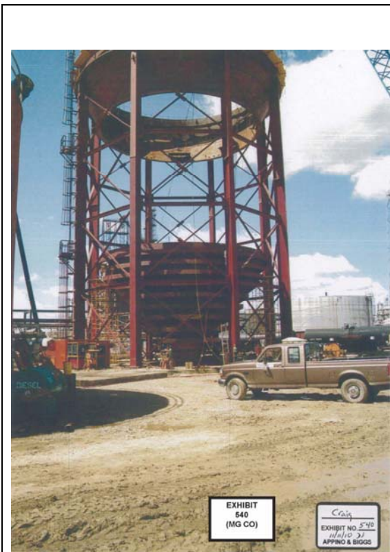
Fig. 7. R. 35, Ex. 540. Coke storage silo being constructed in place on land at the fertilizer plant.
