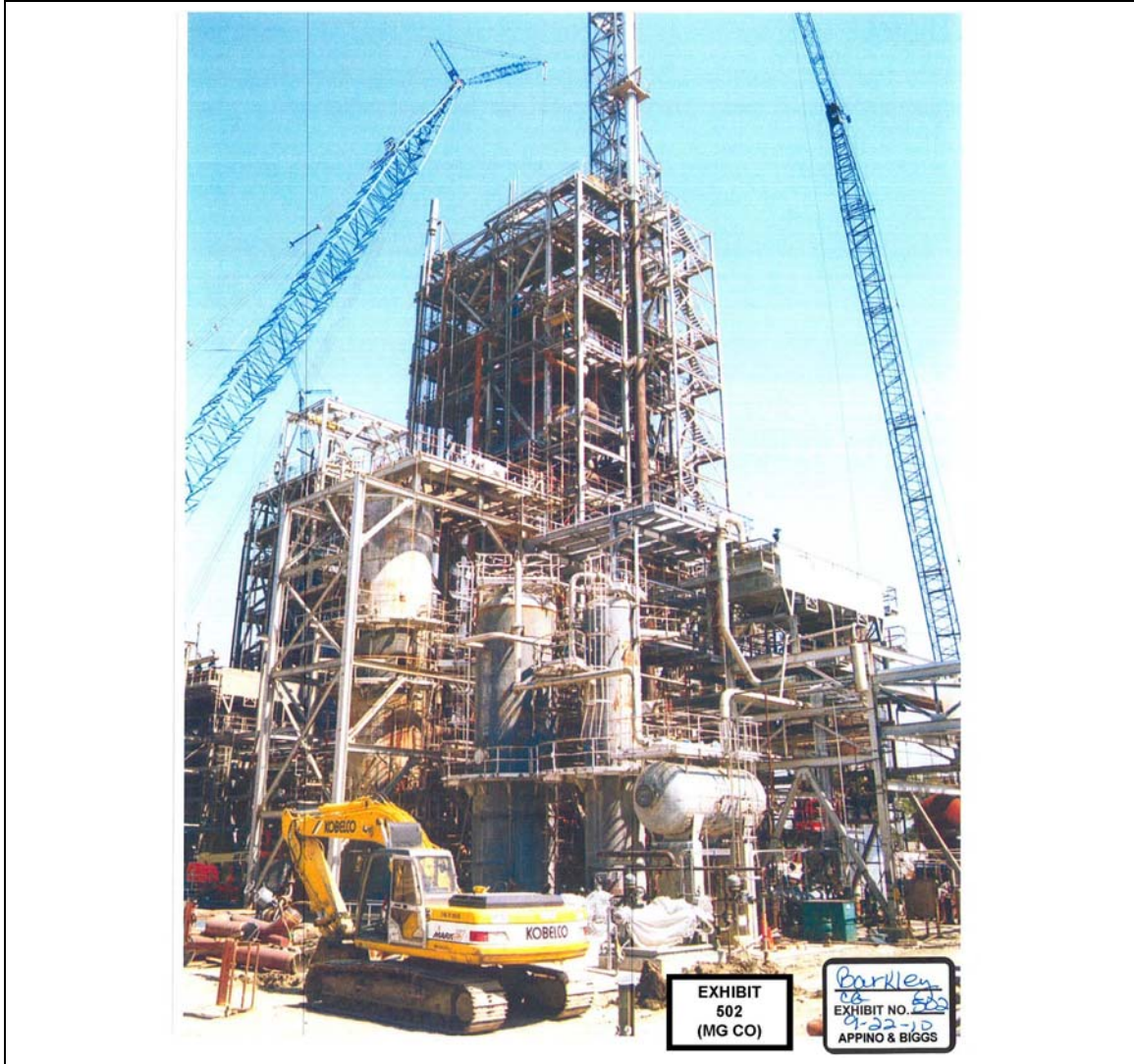
Fig. 3. R. 35, Ex. 502. Main gasifier superstructure (larger structure, background) and gray water system (foreground), under construction.
